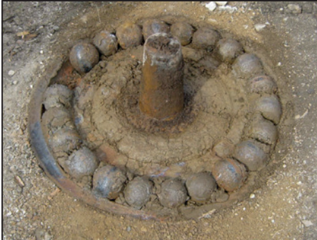
The base of the existing pintle bearing as seen when the bridge was removed for replacement in 2011.
