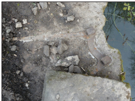
The lock gate anchor strap revealed.
