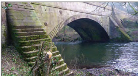
Vegetation clearance has enabled a full view of Jessop's aqueduct across the Derwent, including the huge buttresses that he had to put in after the structure's partial failure in 1793. Photo: Hugh Potter
