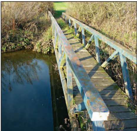
The footbridge across the River Erewash at the site of the aqueduct.
