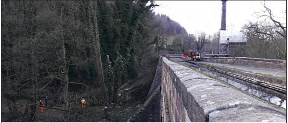
The DCC tree team at work below the aqueduct. with DCC Allroads digging for leaks on towpath by Leawood Pump which itself is having roof repairs.
