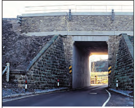
Even modern concrete was no defence against subsidence as can be seen from the displaced left-hand section.
