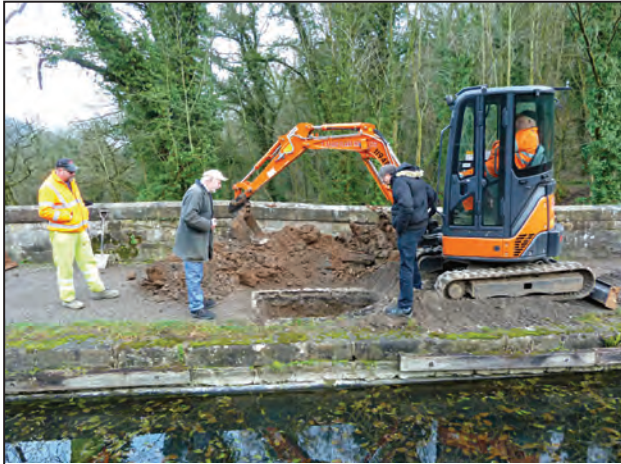
Simon Stoker (left) and Chris Broome “look into” a deep trench dug by DCC’s AllRoads team in the search for the elusive leak(s).
