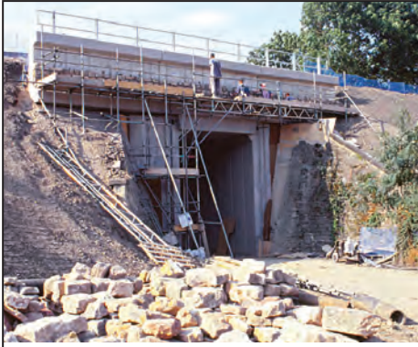
Replacing the historic bridge with a higher concrete structure. Photos: Ian Handley
