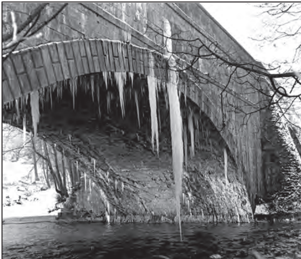
The installation of the liner in the 1980s certainly cured the worst of the leaks – as evidenced in this photograph by the late Frank Rodgers of the effect of the leaks in a very cold winter prior to the its installation. The problem leaks today are from under the two smaller side arches rather than the main span.
