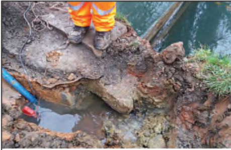
Near the Pump House, a portable pump was used to try to empty the trench dug, through which water was flowing around the stop planks. Note the liner visible under the coping stone and the water movement indicating a leak Photo: Chris Broome
