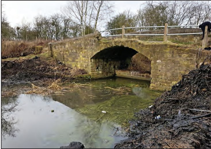
The present sad state of Portland Basin Bridge.
