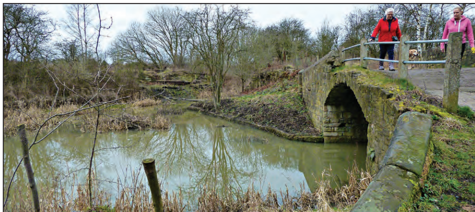
The badly damaged entrance bridge to Portland Basin, recently rechristened 'Humpy Bridge' by locals, is the subject of a funding bid, results of which were awaited as we went to press.
