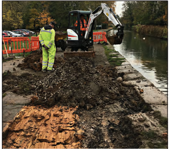
At the Cromford Wharf leak site, a trench was dug and backfilled with puddle clay until . . .
