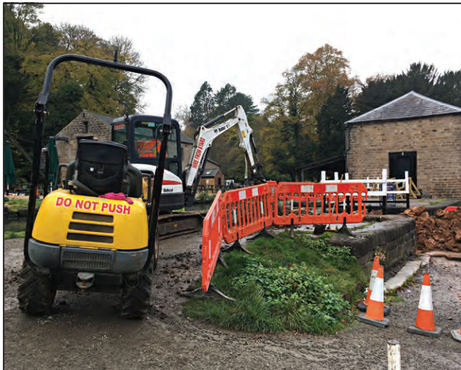
The wall between the cones and the puddle clay had been leaking for some time and partly staunched with sandbags. Not only was the canal leaking, but a 'French drain' designed to run any such water into a land drain had become blocked, causing the leaks through the stonework.
