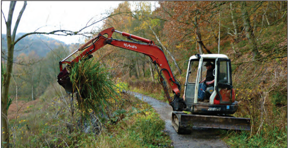
Work was aided by the ability to dump the spoil down the embankment alongside.
