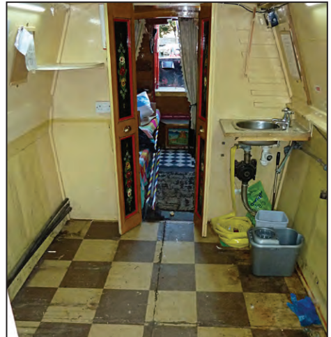
Planning ahead. In February, during the 'quiet' time before the start of season this year, the galley floor was adapted so that the hull beneath it could be readily inspected by the MCA this November. The kitchen was cleared, the four large original (and heavy!) steel base plates were removed, then cut so that they could be easily lifted in future without demolishing the kitchen again. Here, the galley is cleared and the plates await lifting.
