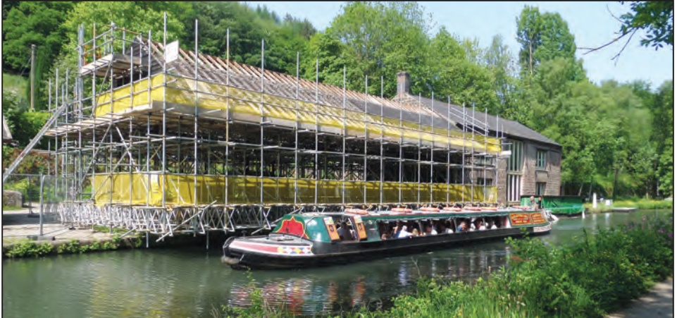
Birdswood passes the impressive scaffolding of the Wharf Shed canopy from which most roof tiles have been removed.
