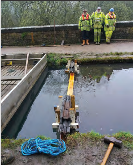
Stop planks at Leawood Aqueduct with weights to hold them prior to securing. Photo: Mike Kelley
