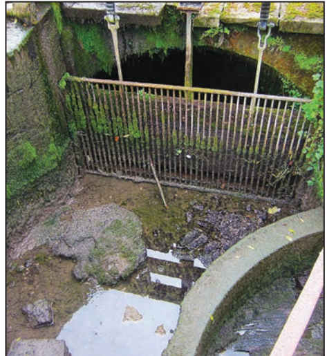
Existing by-wash sluice gate, which forms the overflow weir maintaining a constant head for the new flow control.
