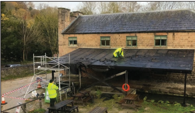
Arkwright Society removing the 30-year-old felt covering in November 2017 to prevent it getting blown off and causing injury.
