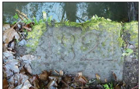
The date 1821 carved into the stone coping where the water from the mill yard enters the feeder arm of the canal.
