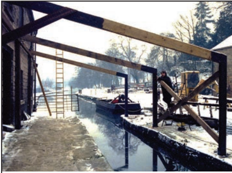
The framework for the new canopy begins to take shape in January 1985 with additional 'cross' strats as requested by DCC.
