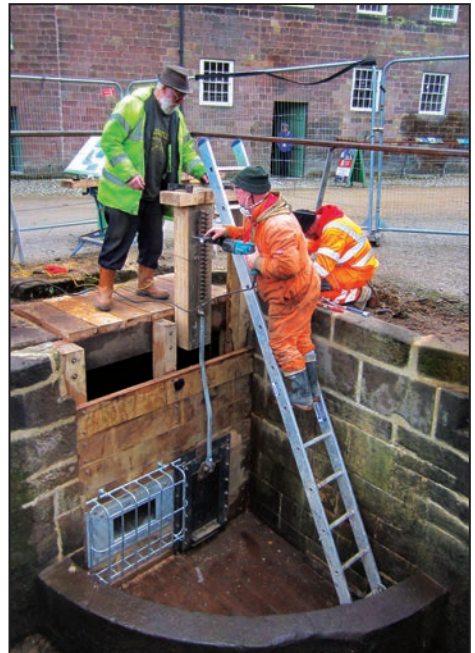
Installing the paddle rack gear. The orifice plate and weed screen can also be seen.
