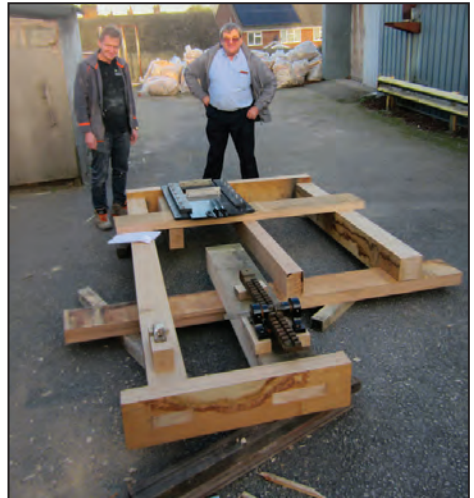
The new water control sluice for the canal feeder at Cromford Mills being trial assembled in the joiners works in Somercotes. It should have been installed at Cromford by the time you read this, and will hopefully restrict flows into the canal in times of flood and make water level management much easier. Looking on are Peteris, a Latvian carpenter who made the frame (left), and Bob Mitchell who supervised the work. Photo: John Boucher
