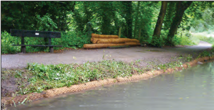
The finished job; in a few weeks nature will have taken back over.
