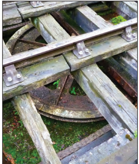
The huge pulley wheel in its pit (note rotten timber) at High Peak Junction.
