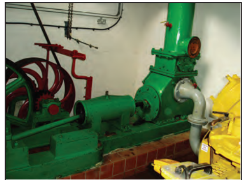
The original 1894 reciprocating pump. No makers marks have been found.
