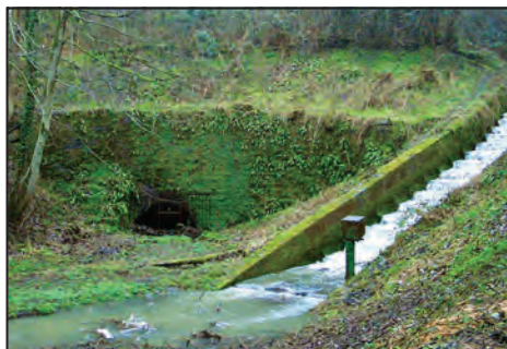
A good flow of water coming from the Butterley Park feeder at the eastern portal of the tunnel.
