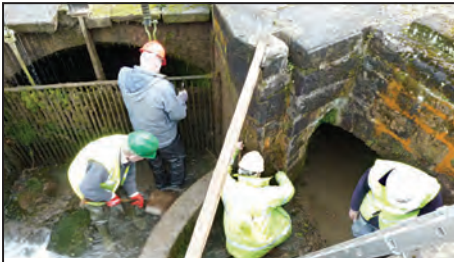
The FCC team clearing the weir pit in Cromford Mills. The culvert to the canal is to the right (the groove in the far stonework can be seen) and the overflow to the river is top left.
