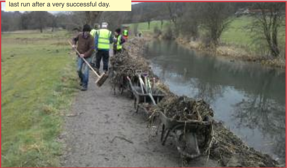
Above: A steady stream of barrows forming the convoy transporting the reeds up to the tipping area at Cromford Wharf. Below: Tiding up the towpath prior to the last run after a very successful day.
