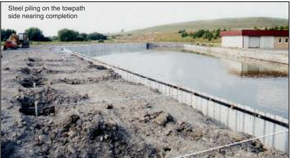
Fixing shuttering prior to pouring concrete to build up the offside wall
