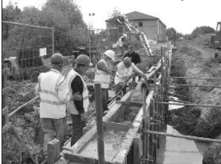
Pumping the concrete from the Chrysalis Way car park to the far end of the shuttering
