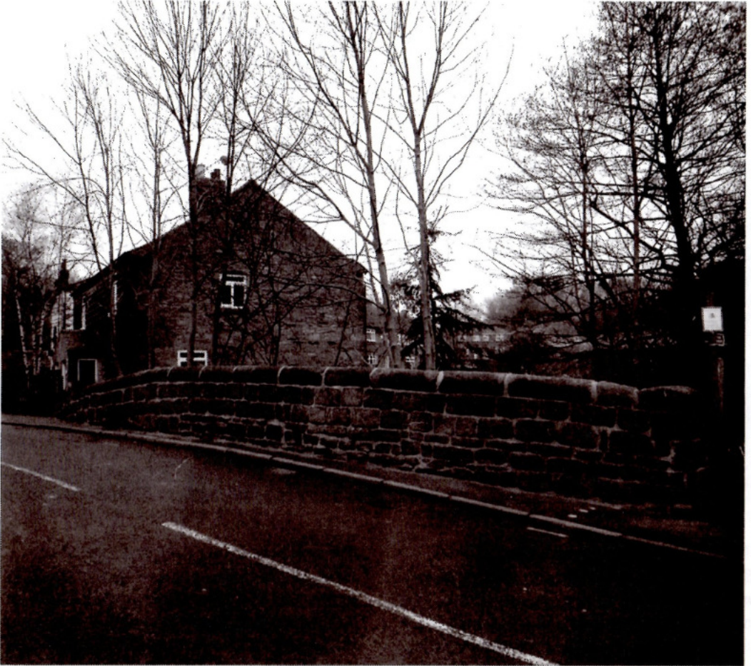
The job done - walls repointed and a few holes in the road
