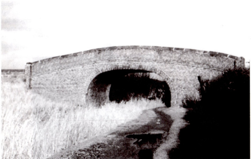
This photograph was taken in the 1960's and depicts the bridge with its flat arch, when it was in relatively good condition.
