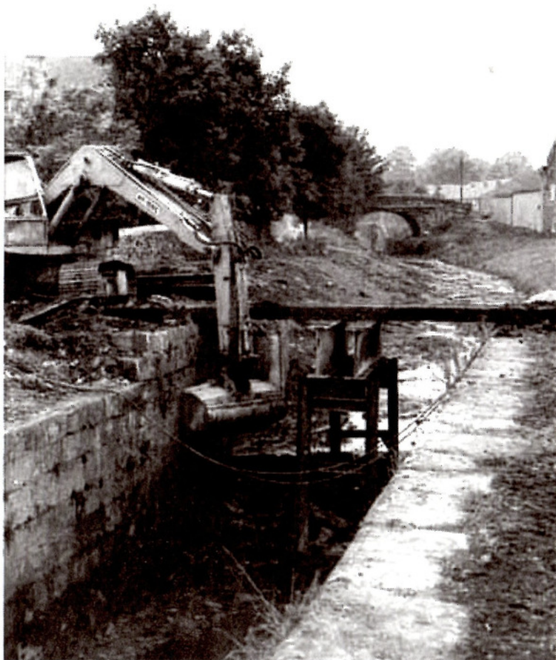
A closer view of the work at Lock 4 with Bridge 37 in the background.
