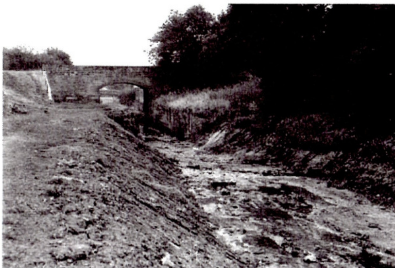
A muddy mess above Lock 2, the sill of which has been removed, and Bridge 36.
