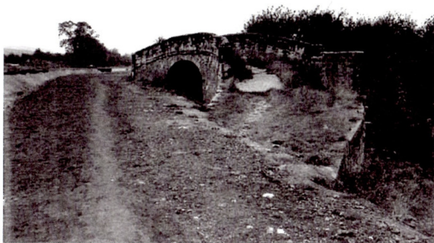
The Pinxton Branch junction bridge is left 'high and dry', barricaded off by dredgings from the huge channel to the left.
