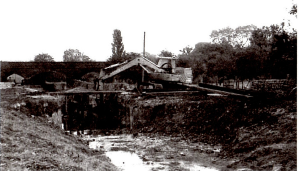
Work pauses for the weekend at Lock 4 where the concrete sill has been removed but the remains of the central sluice are still in place. In the background is the Erewash Valley line railway bridge.
