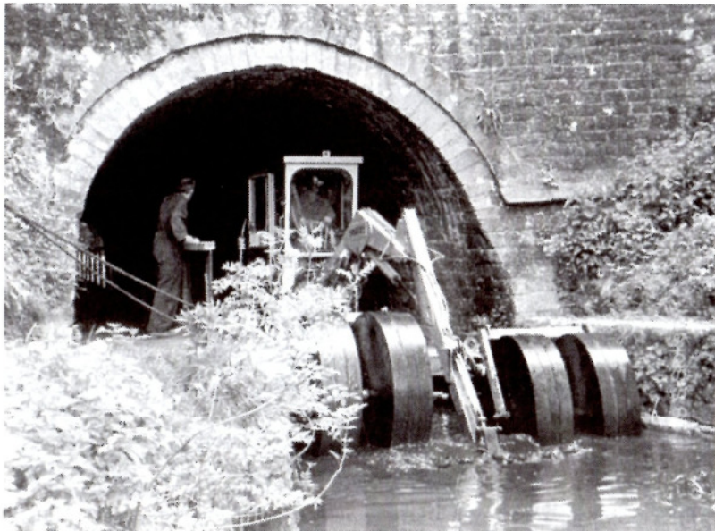
Dredger emerges from Gregory Tunnel into Gregory Dam. Considerable rubbish in mouth of tunnel made machine ride up on its wheels.
