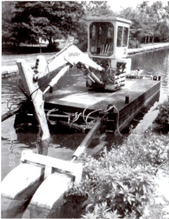
Original long-reach Smalley excavator converted to floating dredger by manufacturer. Very effective. Pontoon made narrower than their standard @6ft 10in to get into drydock and through tunnel.
