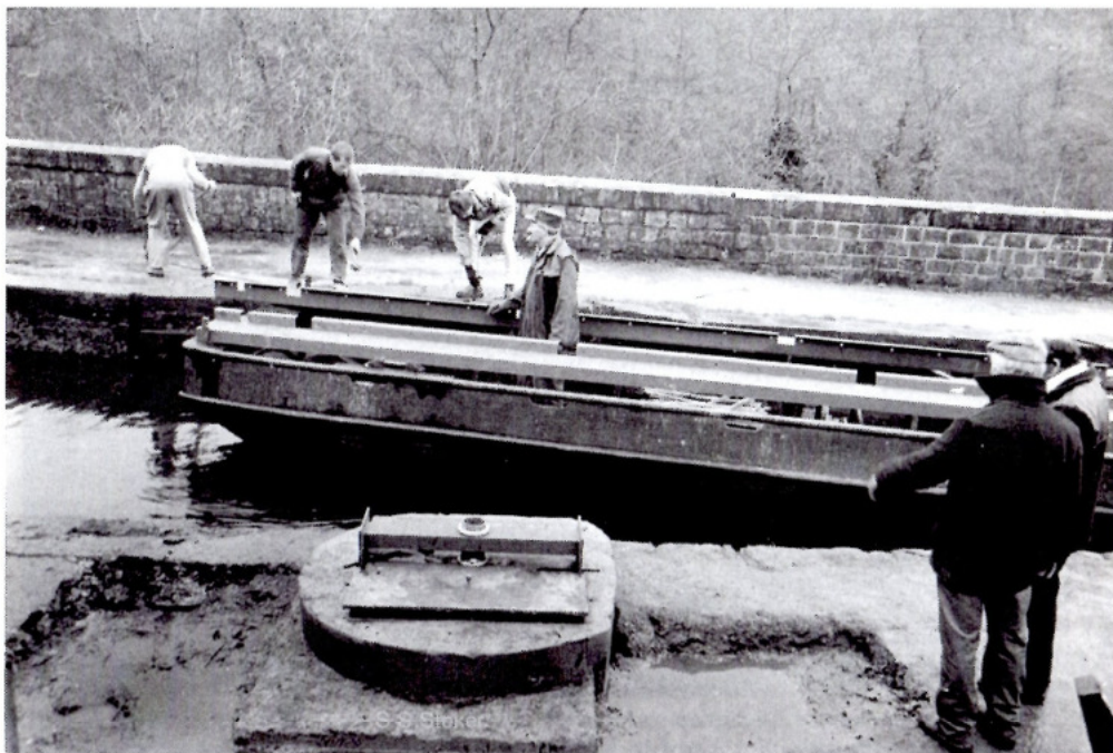
TRANSPORTED by water the 1 ½ miles from Cromford the galvanised sections arrive on our work boat. In the foreground is the completed main bearing assembly on the main concrete base. (The rest was filled later).
