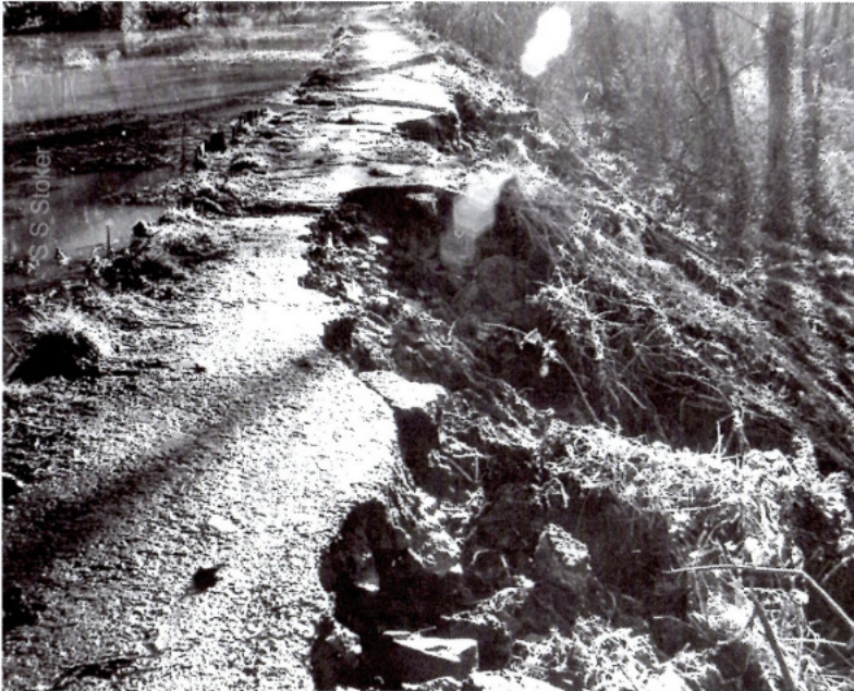
The OTHER point at which the water overtopped the bank on 25 th February 1989. This was about 350 yards east of the first point, roughly 300 yards west of the tunnel. No steel piles were inserted here, with the result that the towpath nearly went completely.
